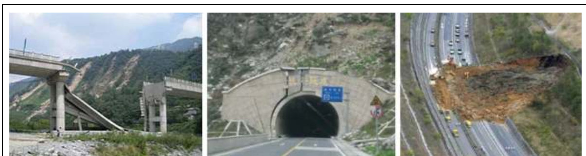
Fig. 01. Examples of traffic disruption due to key network component failures (bridges, tunnels and slopes by Kilanitis, I., Sextos, A. 2019
