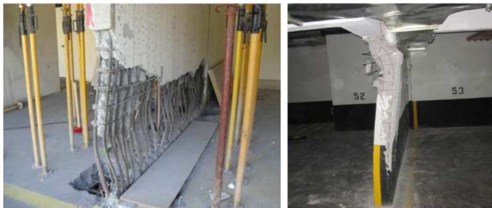
Examples of overall wall lateral buckling from the 2010 Maule earthquake: (a) Alto Huerto building, Concepción (DICTUC, 2010d); and (b) Undisclosed Building B, Santiago (DICTUC, 2010e).
